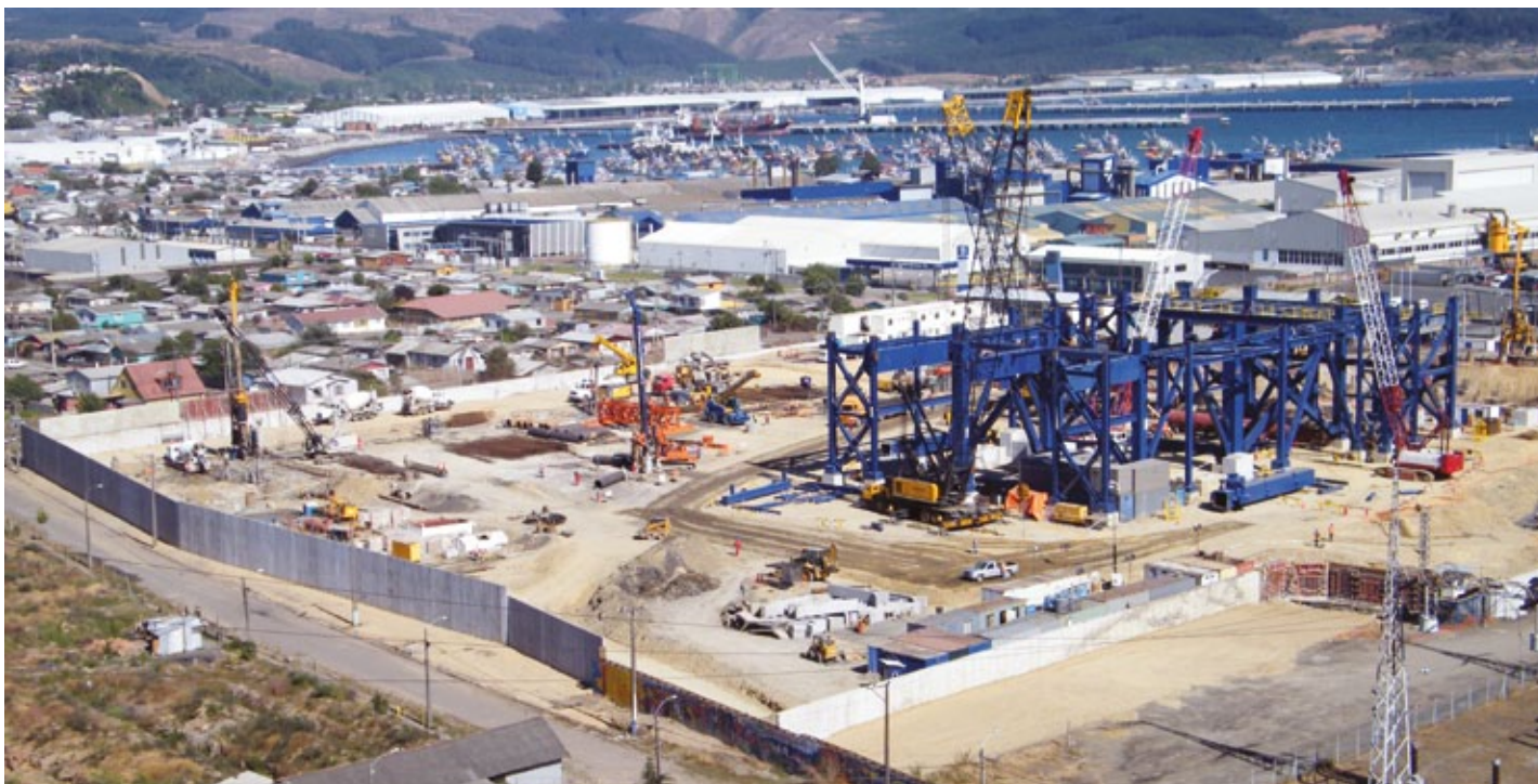
Central Termoelectrica Bocamina II
