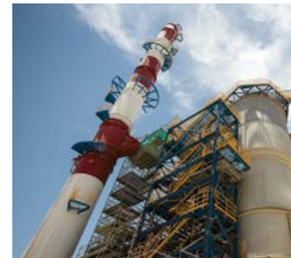
CIVIL WORKS AND ELECTROMECHANICAL ASSEMBLY OF ACID PLANTS 3 AND 4, CHUQUICAMATA MINE OF CODELCO, CALAMA, CHILE
