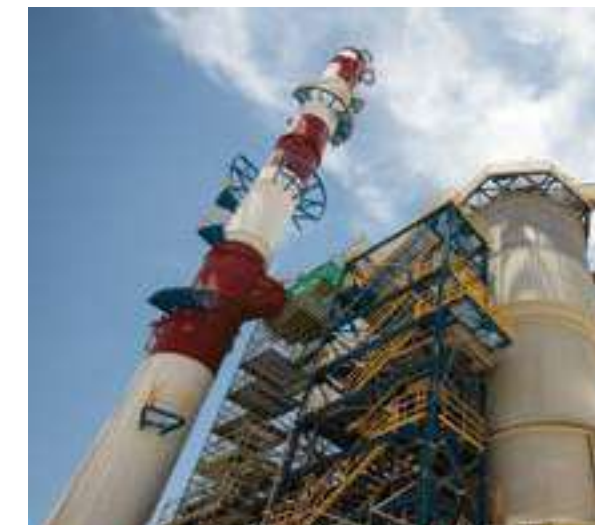
CIVIL WORKS AND ELECTROMECHANICAL ASSEMBLY OF ACID PLANTS 3 AND 4, CHUQUICAMATA MINE OF CODELCO, CALAMA, CHILE
